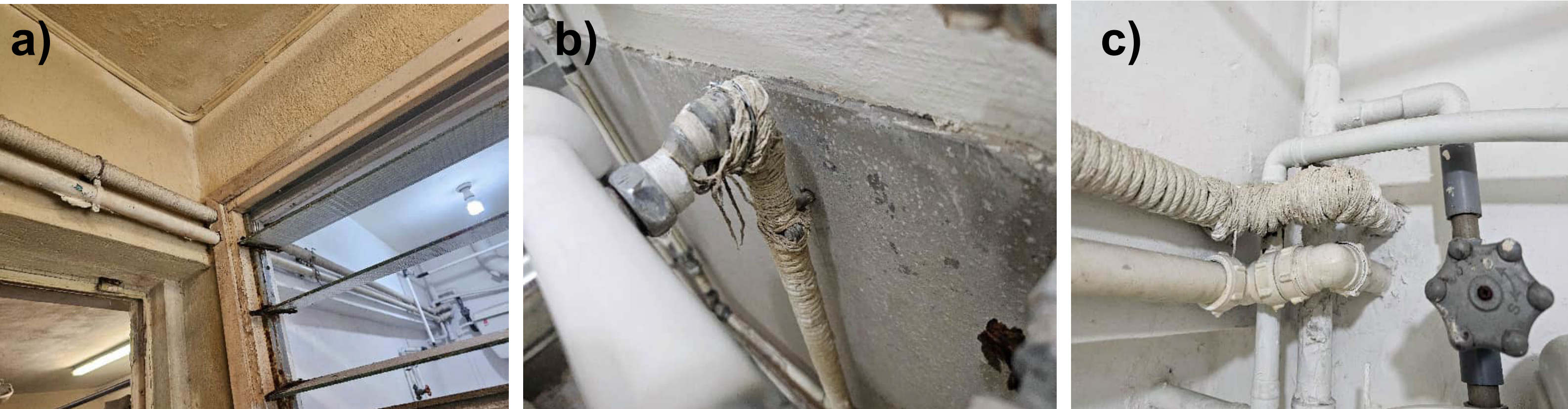
Figure 1. a) Asbestos-containing Rope Lagging in location A; b) in location B; c) in location C at Tung Tau Wan dormitories.
